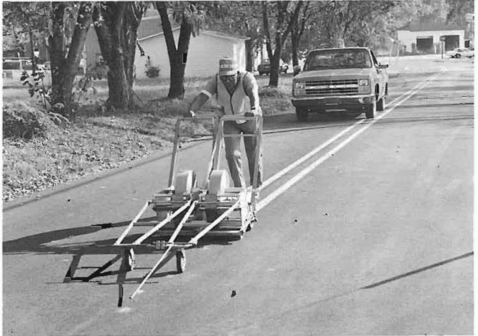
As the special dispenser is pushed down the highway, the tape is placed on the pavement.
